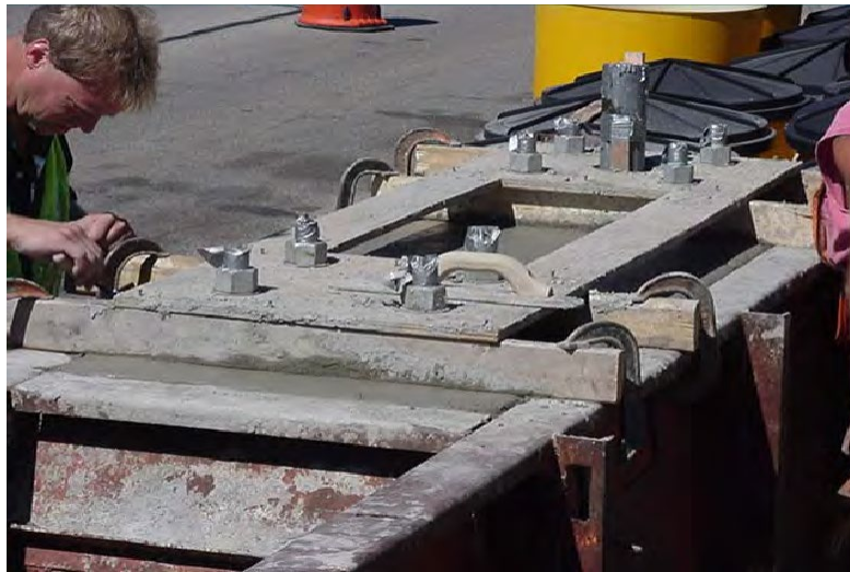
Figure 2. Template Secured to the Forms to Ensure Proper Alignment. Note Anchor Rod Threads Taped to Prevent Contamination by Concrete.
